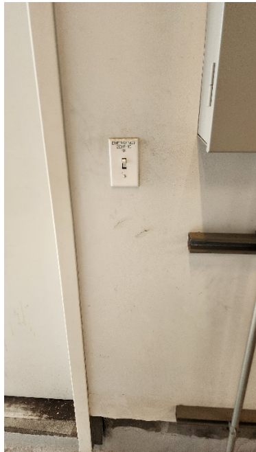
Manual Switch – Boiler Room
