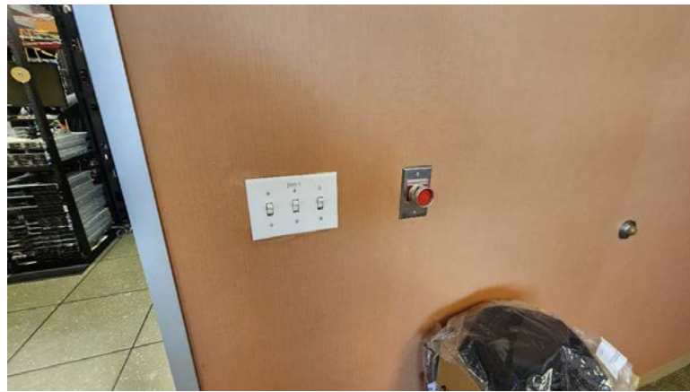
Manual Switch – Open Office
