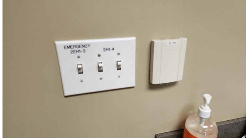
Manual Switch – Conference Room
