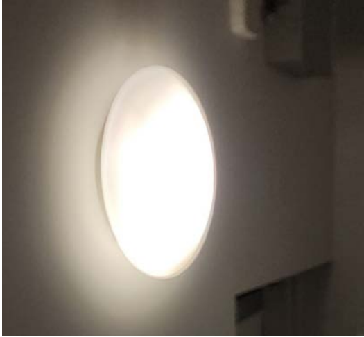
Stairwell Circular (Wall Mount) 2-Lamp 9W CFL
