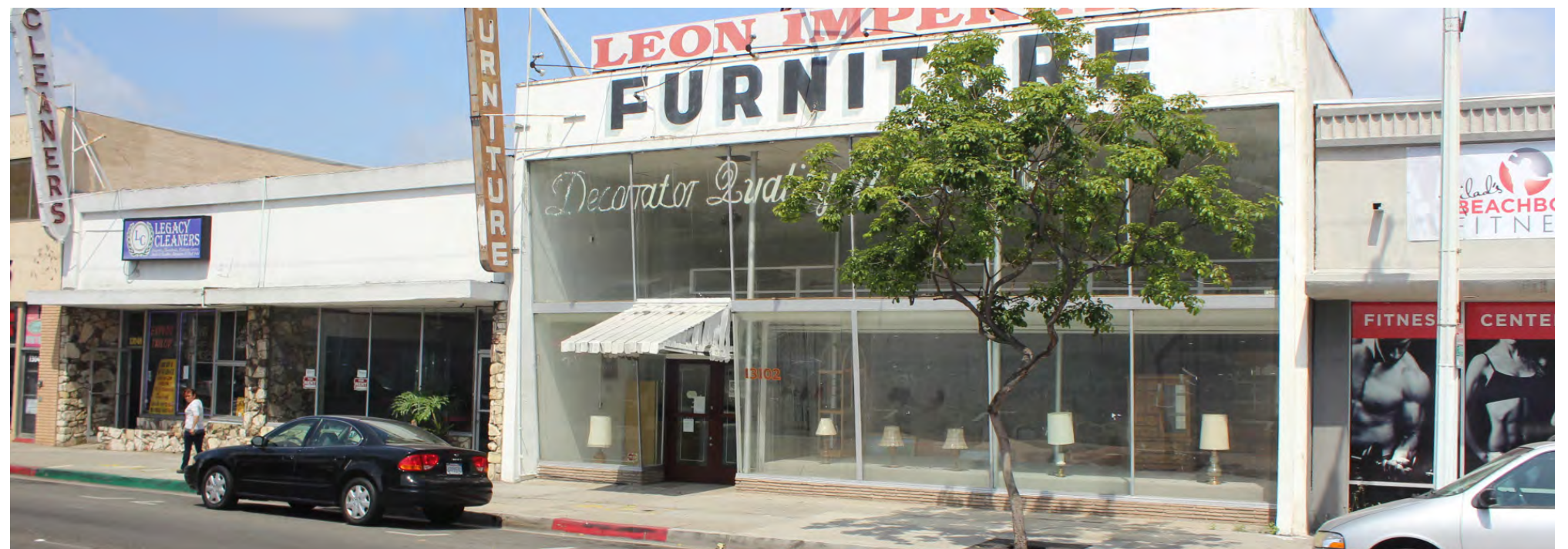
Building facades along Hawthorne Boulevard need to be improved upon, as may vary dramatically in both style and state of repair/disrepair
