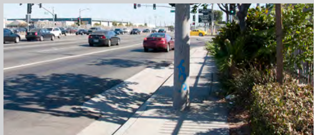
Sidewalks – Sidewalks in the immediate station area are narrow, with physical barriers blocking the path.
